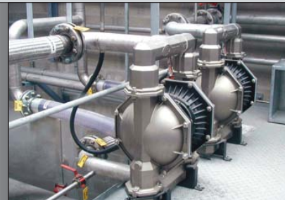
3" stainless steel diaphragm pumps installed on a bulk transfer process.
