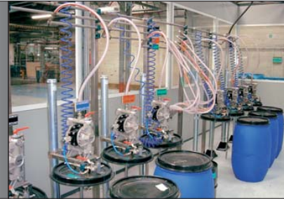
1/2" diaphragm pumps installed in a colouring process
