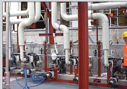
2" stainless steel diaphragm pumps assembled with PVDF pulsation dampeners used to download hydrofluoric acid
