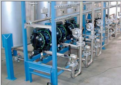
1 1/2" aluminium diaphragm pumps installed to feed a chemical reactor.
